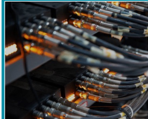
Structure Cabling Systems
