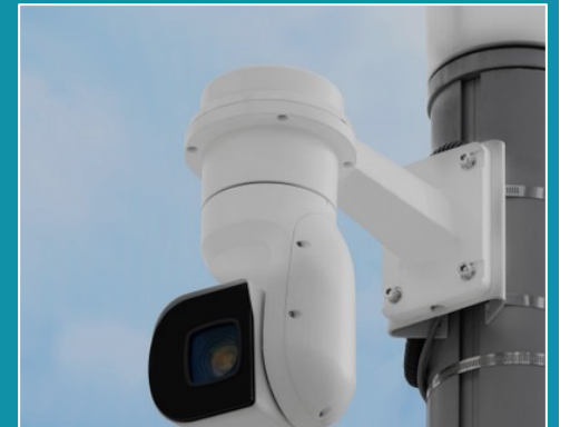
Surveillance & Public Security Systems
